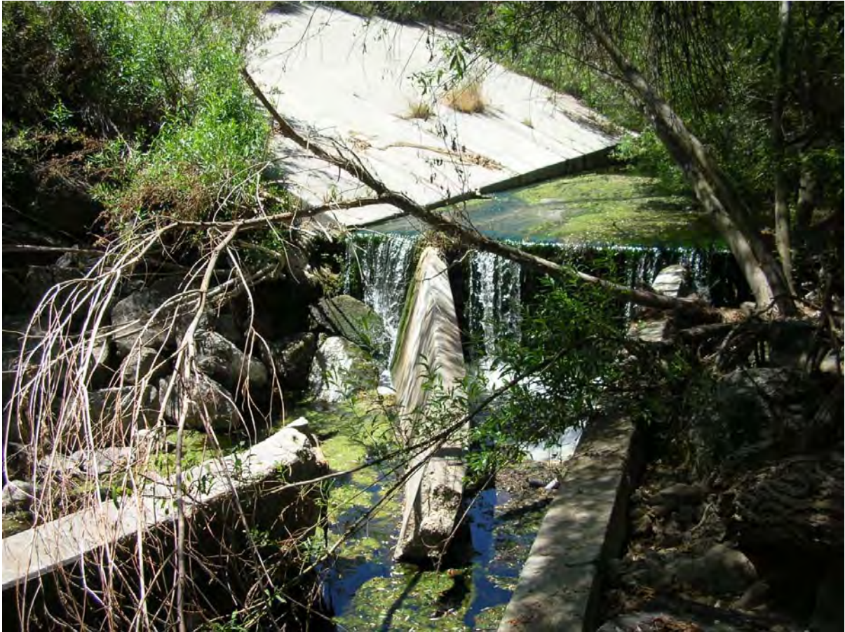
Looking upstream at approximate Station 18+59 – Failed cut off wall and vertical drop in channel invert.
